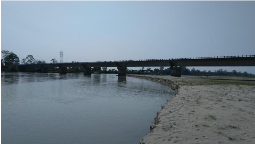
Fig No: 9. Showing Bank bridge connected between Namsai and Mahadevpur. Source: Shelf Click
