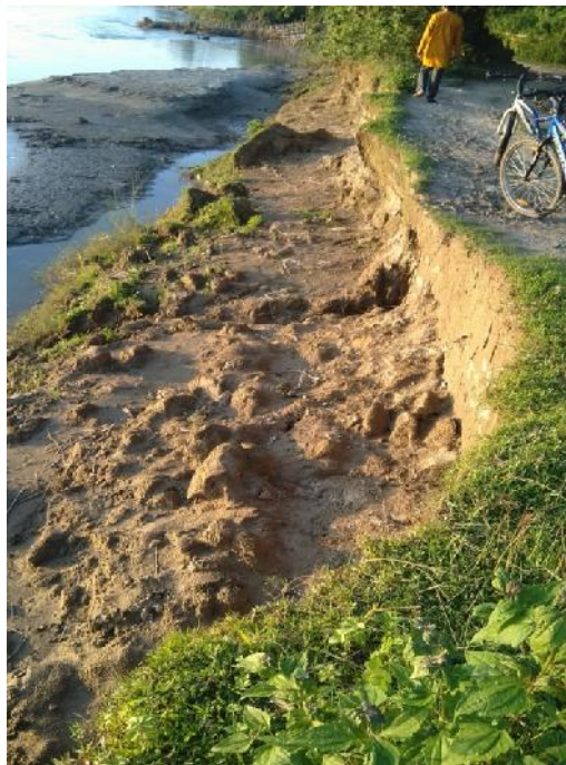
Image No 13: Showing erosion of road of Kharibari village in Namsai Circle.
