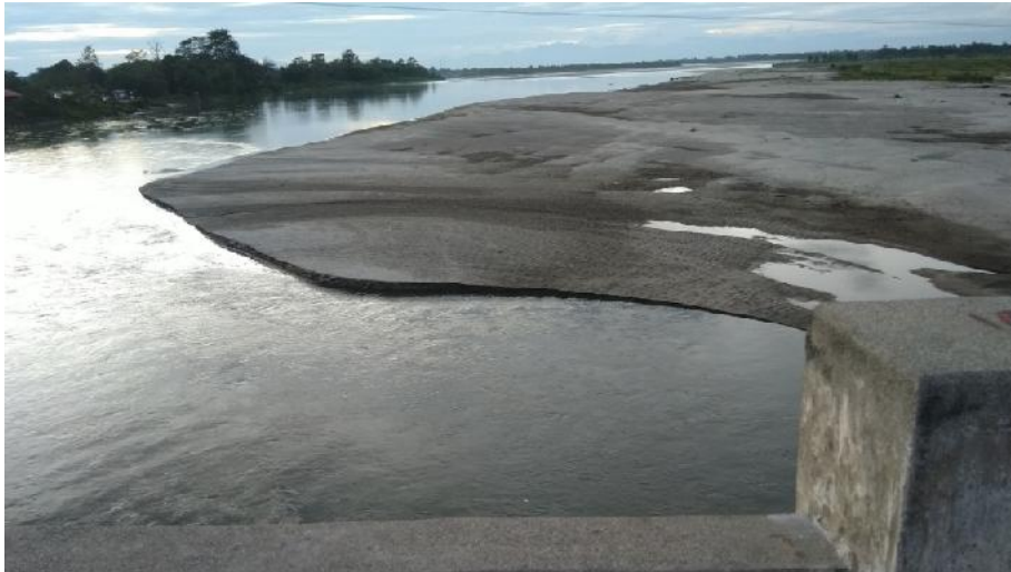
Fig No: 4. Silt Deposition in Dihing River channel between Mahadevpur and Namsai Circle. Source: Self Click
