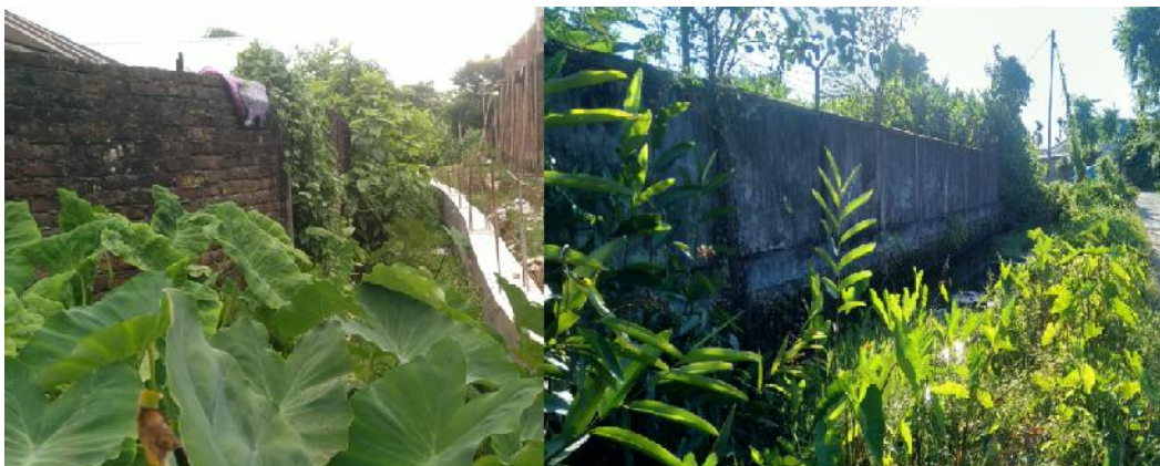
Fig No: 7. Block drain in Namsai Circle. Source: Shelf Click
